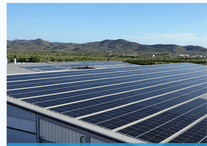
5MW photovoltaic power station project in a factory in Shaoguan
