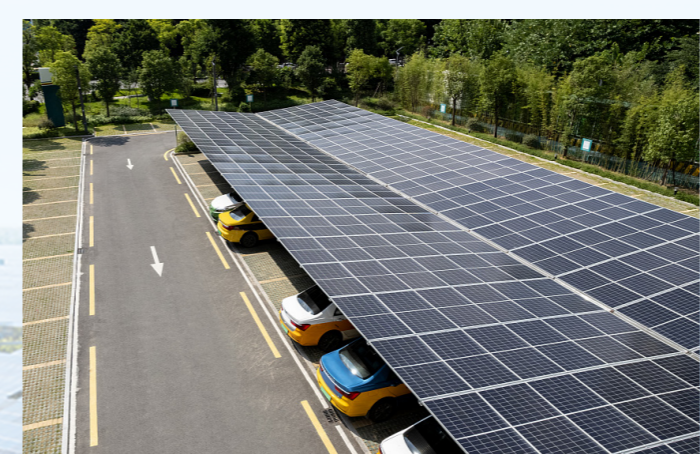
A company's parking shed 200KW photovoltaic power station project
