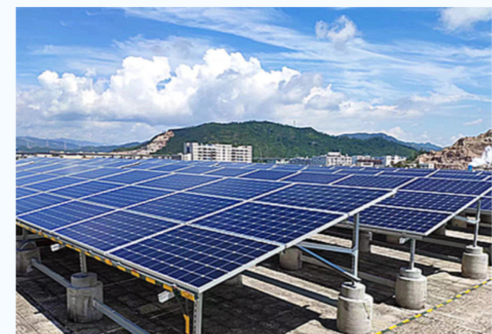
800KW photovoltaic power station project of a school in Guangdong
